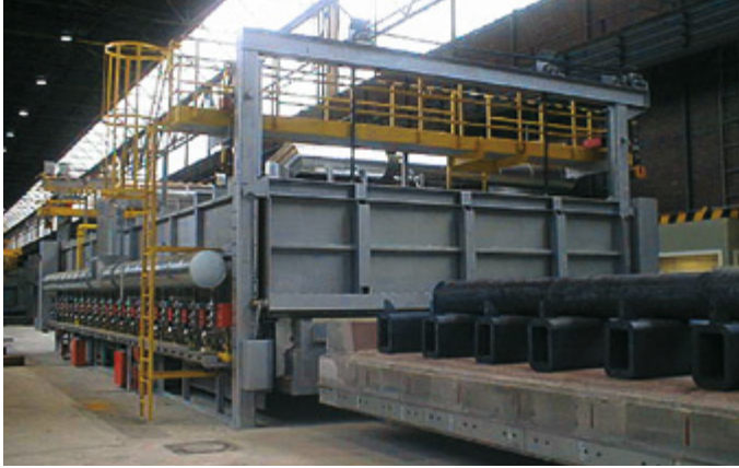
Metallurgical industry: bogie hearth furnace
